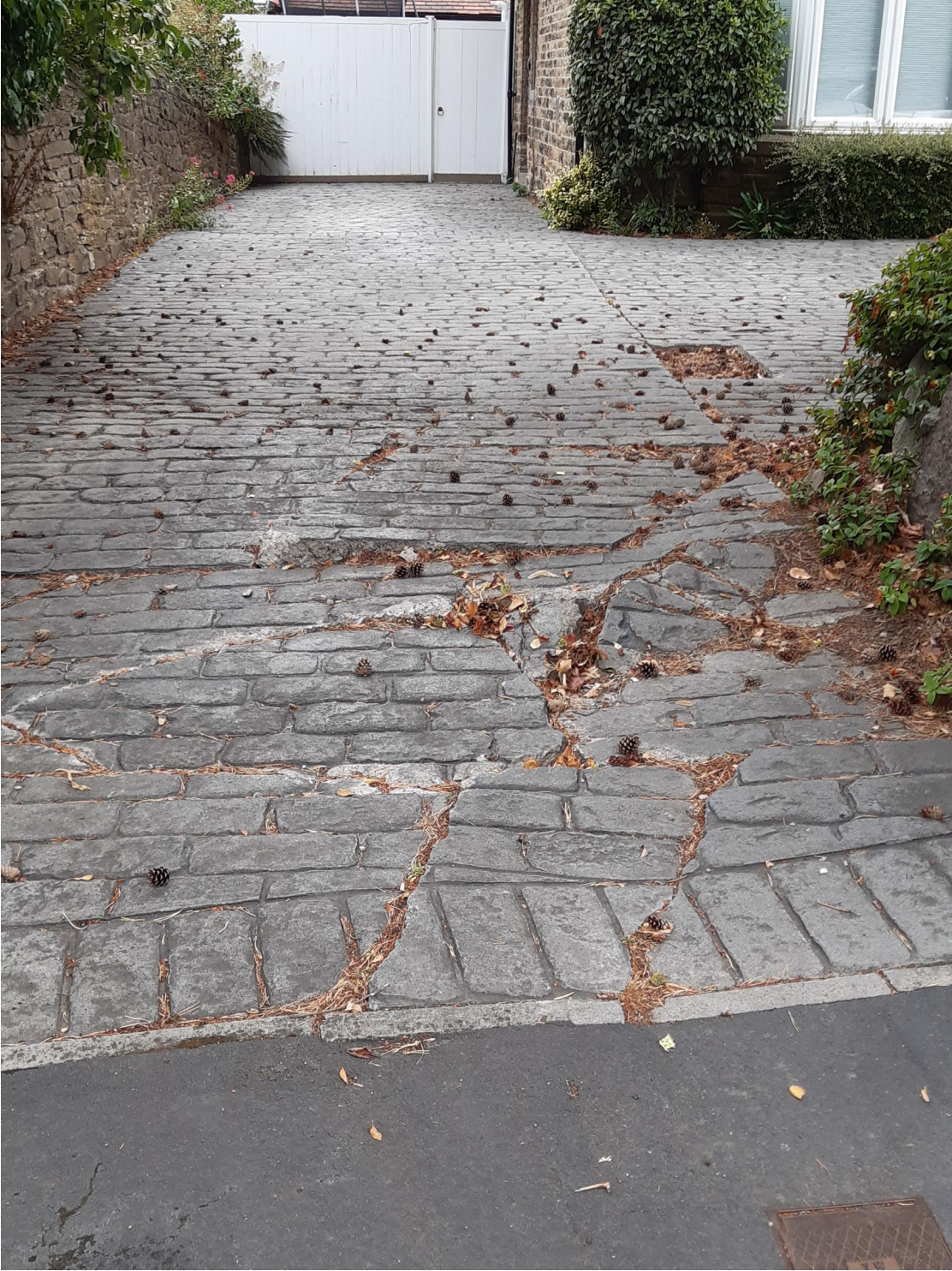
Image of damage to drive.
